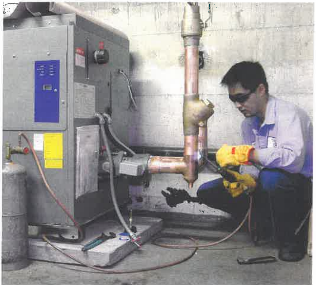
An ACA Denver Boiler technician completes connections for a Laars Pennant boiler/volume water heater in an apartment building in downtown Denver.
